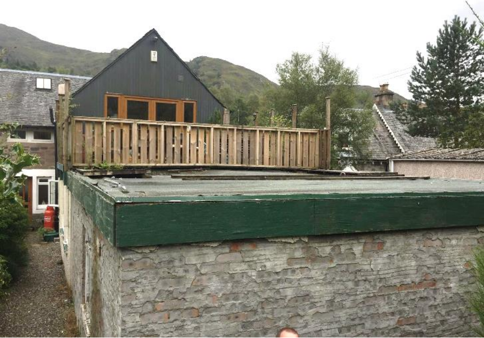
Figure 4 Photo taken from behind the garage looking over its roof to Braehead Cottage upper level with balcony and original rear elevation behind, to the side.
