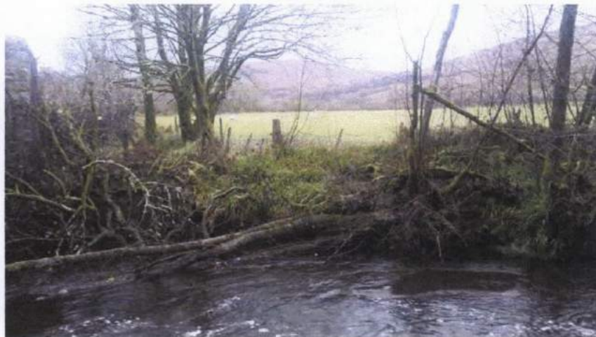
Plate 11 – Fallen mature tree at the A815 road bridge (upstream side).
