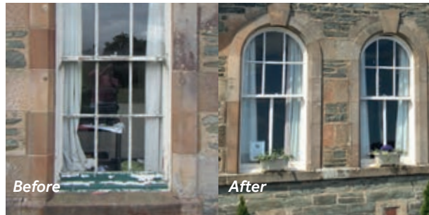
Blairmore Community Hall Restoration of Windows – Retaining an important feature of this listed building.
