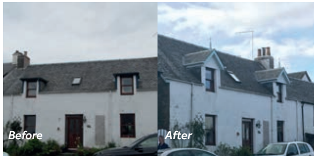
Gartmore Restoration of pitched slate roof dormers. Building on other enhancements in the village that have benefitted from our grant.
