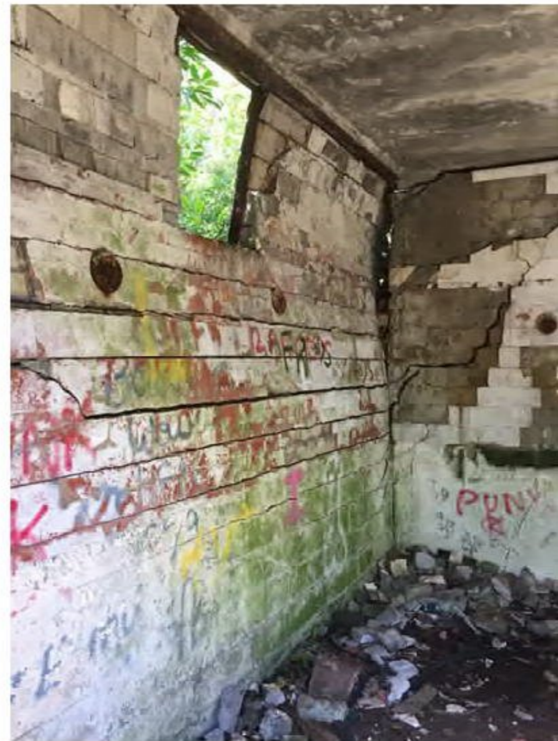
Photograph 23 – internal view of west wall in north block Showing failure
