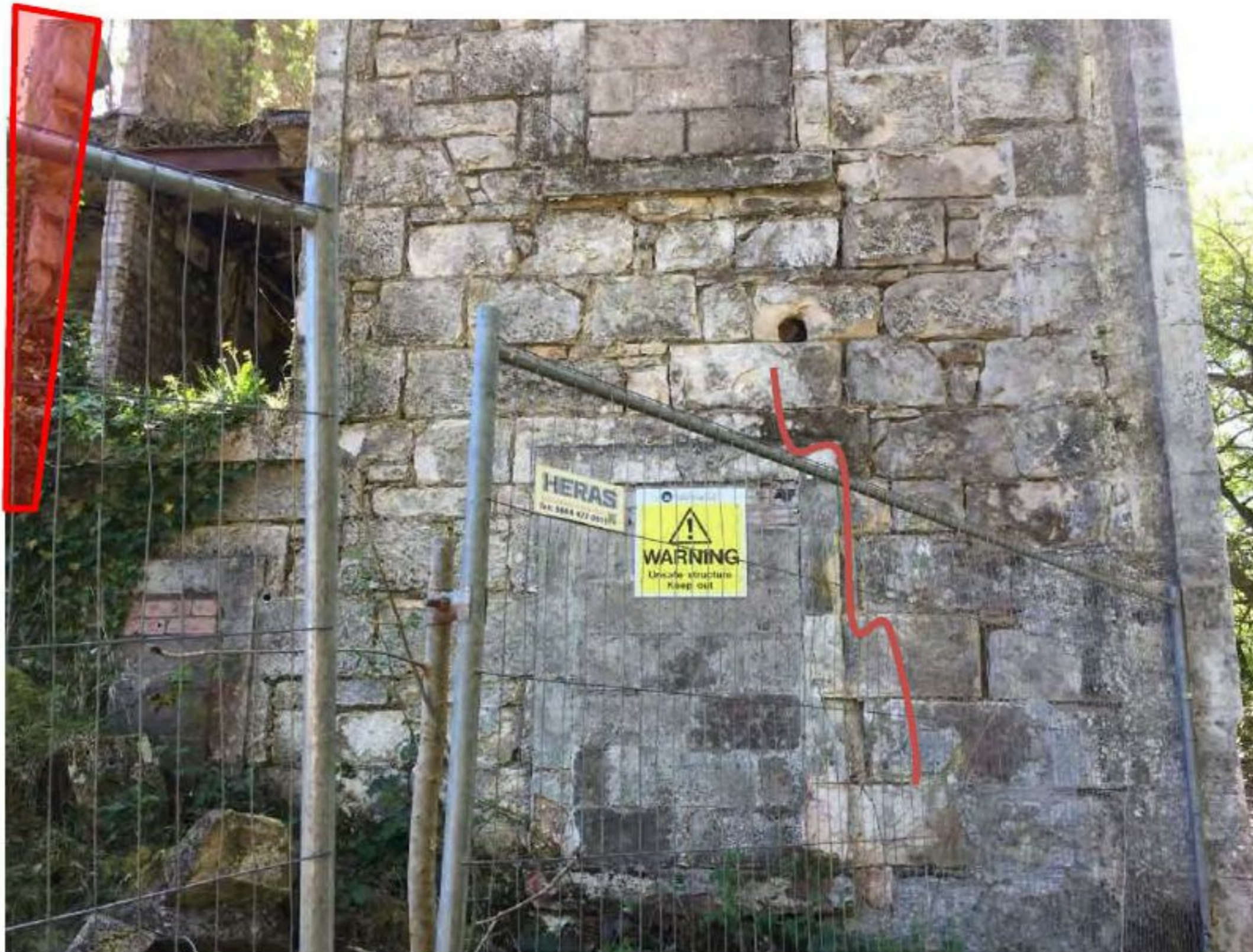
Photograph 9 – North Rear Elevation West low level Priority down takings highlighted red, cracks highlighted in orange.
