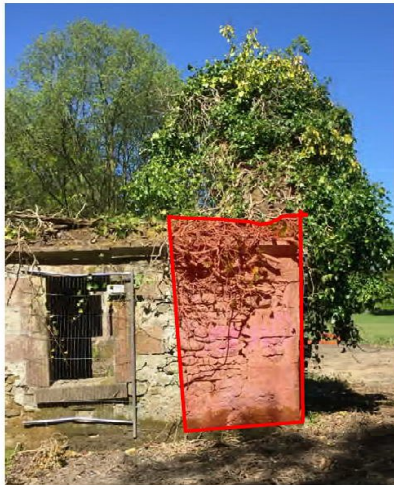
Photograph 21 – East end of South elevation of south block Showing bulging wall and down takings in red
