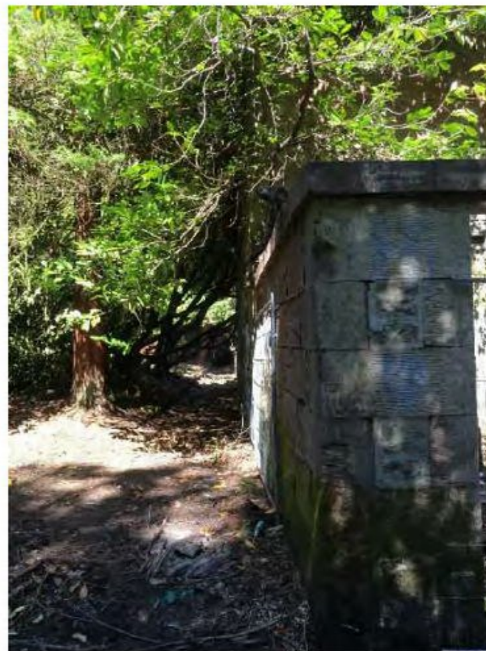
Photograph 26 – West wall of rear section Showing unstable walls and trees.
