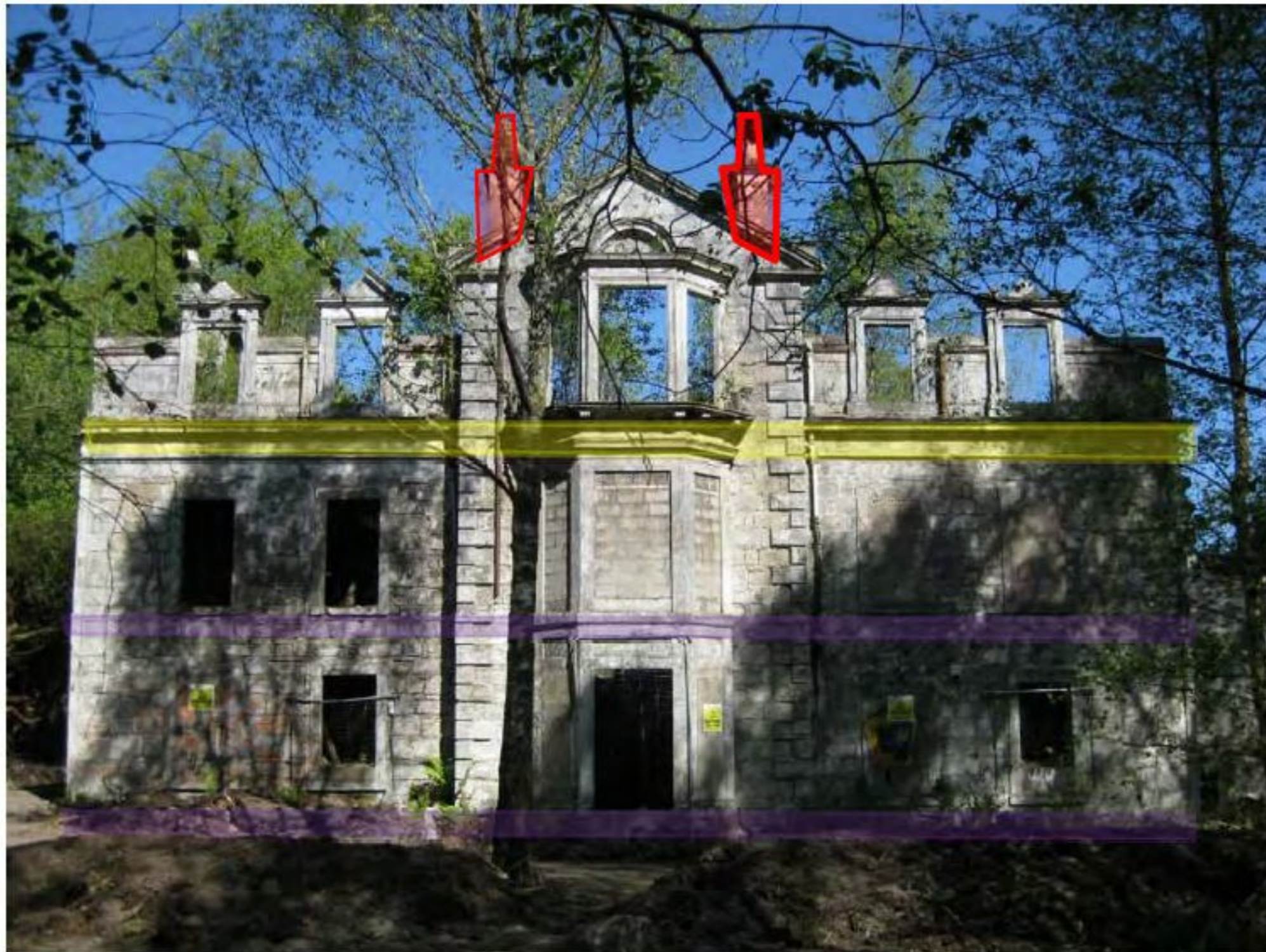
Photograph 5 – South elevation Down takings for safety highlighted red, unstable floors behind highlighted yellow and missing timber floors highlighted in purple.
