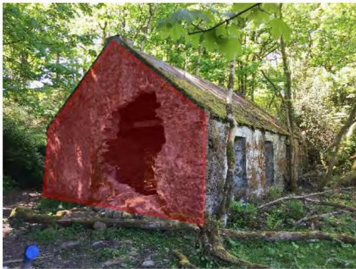
Photograph 27 - South wall showing collapse Priority down takings for safety highlighted red.
