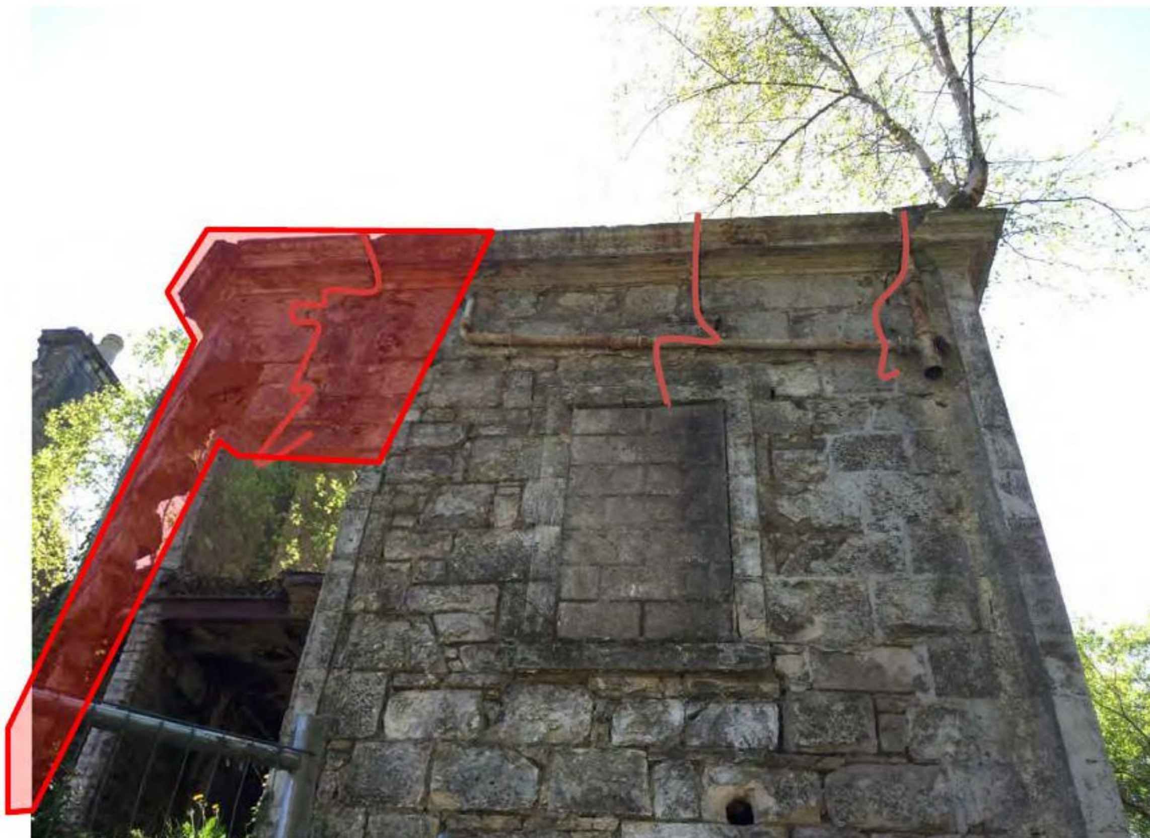
Photograph 10 – North Rear Elevation West high level Priority down takings highlighted red, cracks highlighted in orange.
