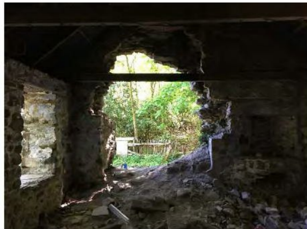
Photograph 32 – South wall, showing collapse.
