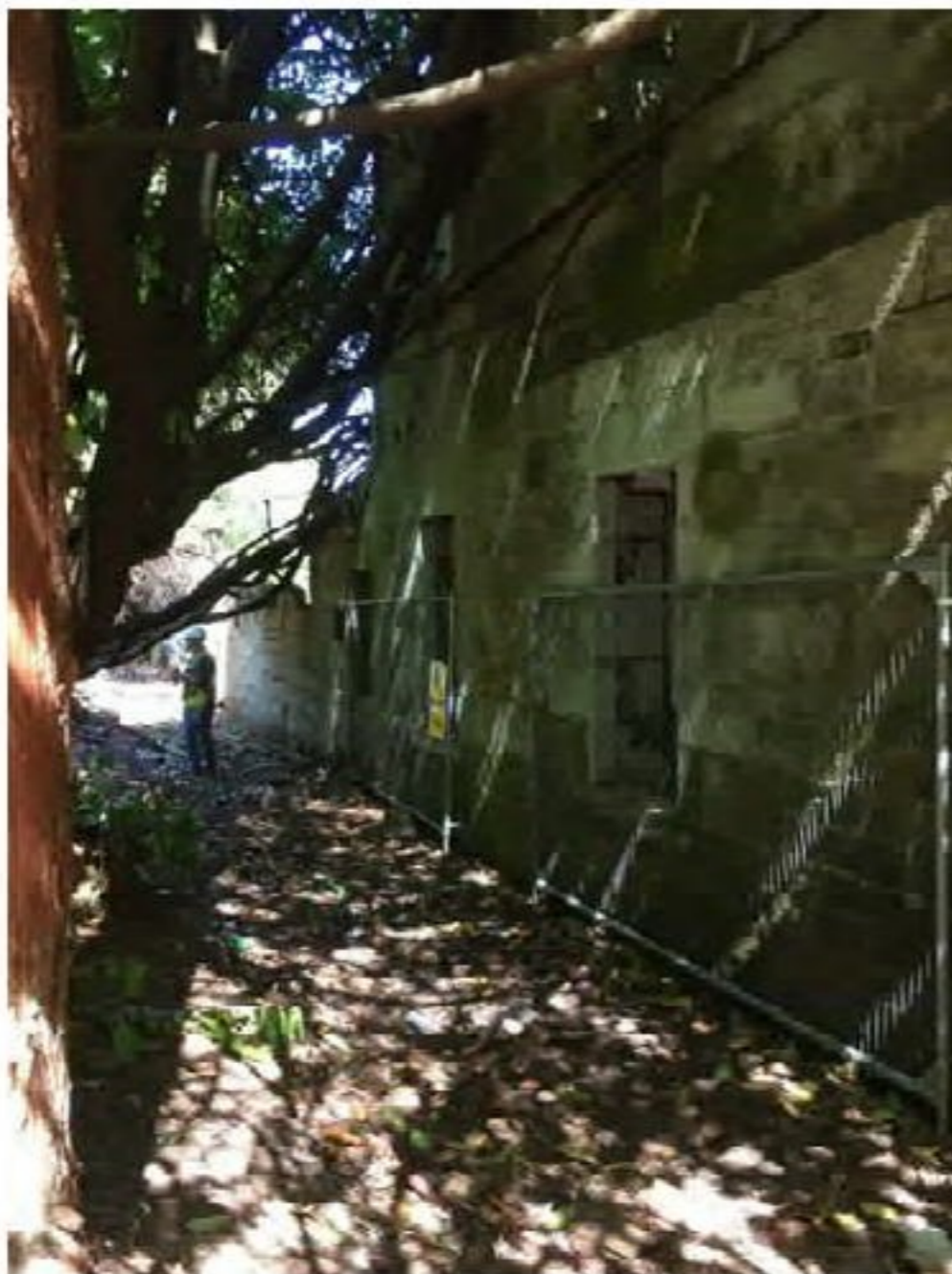
Photograph 25 – West wall of rear section Showing unstable walls and trees.
