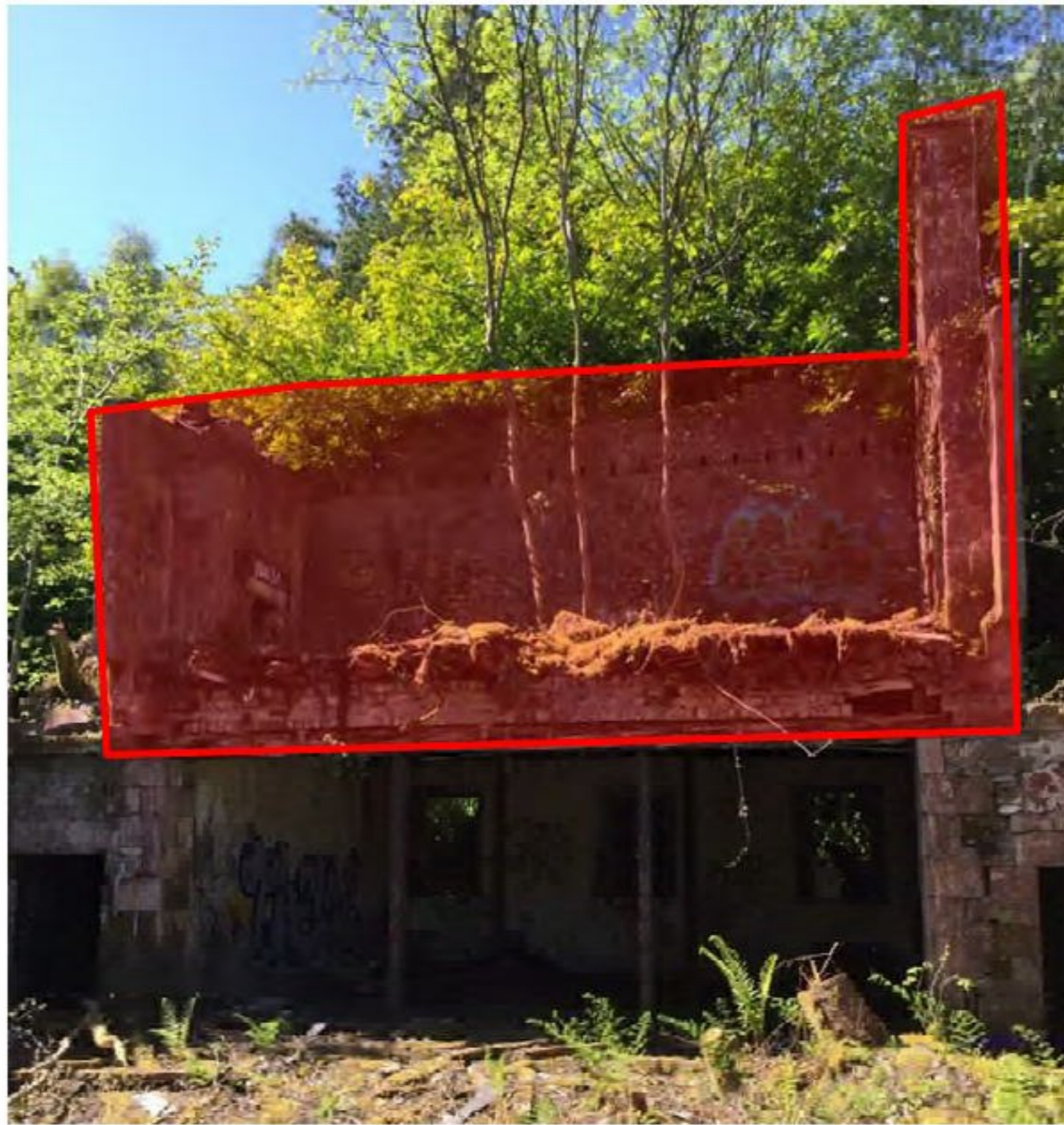
Photograph 24 – first floor of rear section Showing priority down takings for safety in red
