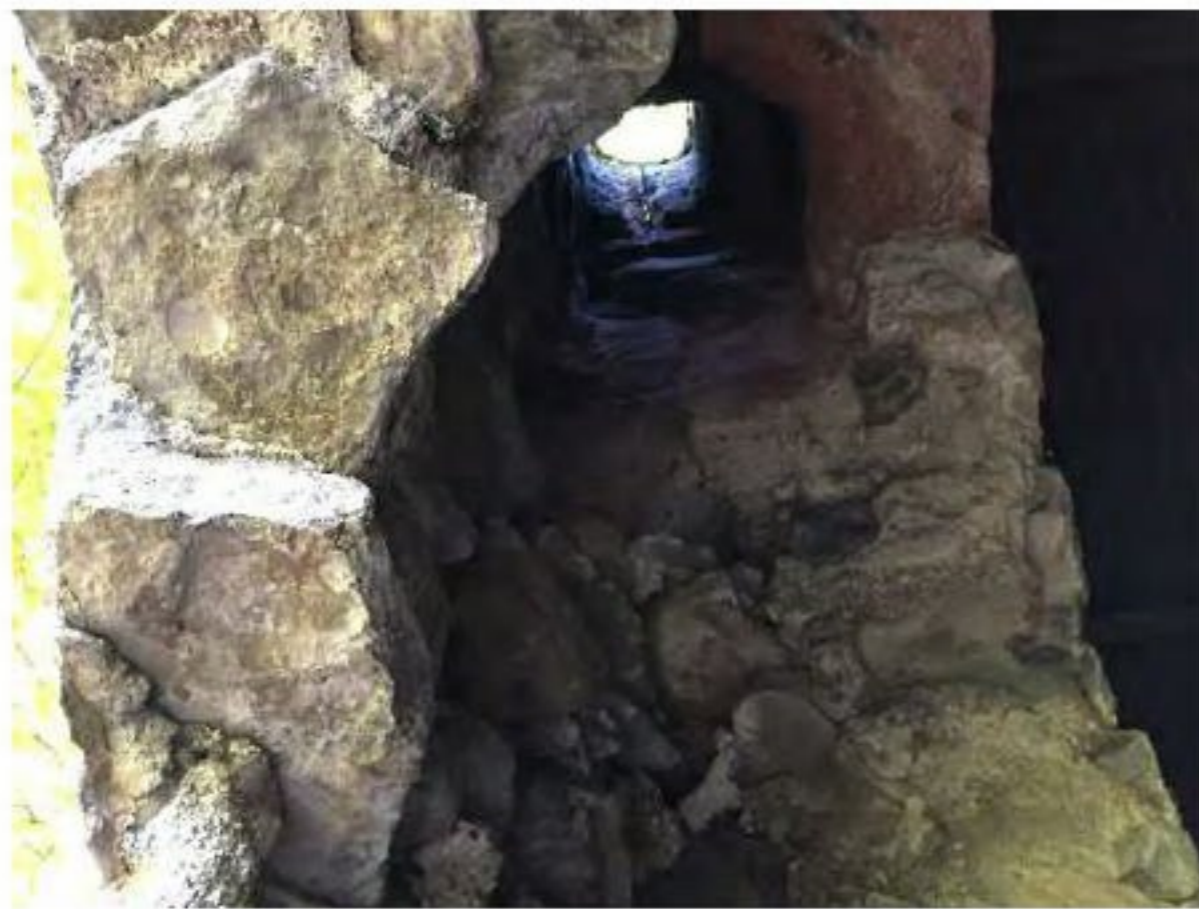
Photograph 29 – South wall, showing unstable flue.
