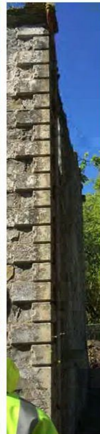
Photograph 12 – bulge in North east elevation
