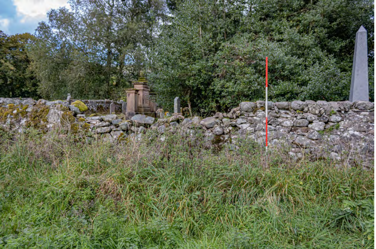
Plate KG14: Kilmahog Graveyard, south boundary wall, detail of damage from the south
