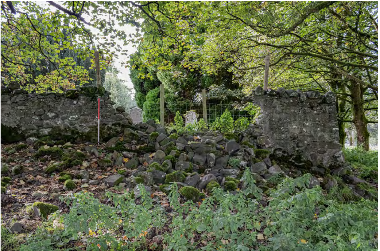
Plate KG13: Kilmahog Graveyard, east boundary wall, detail of damage from the east
