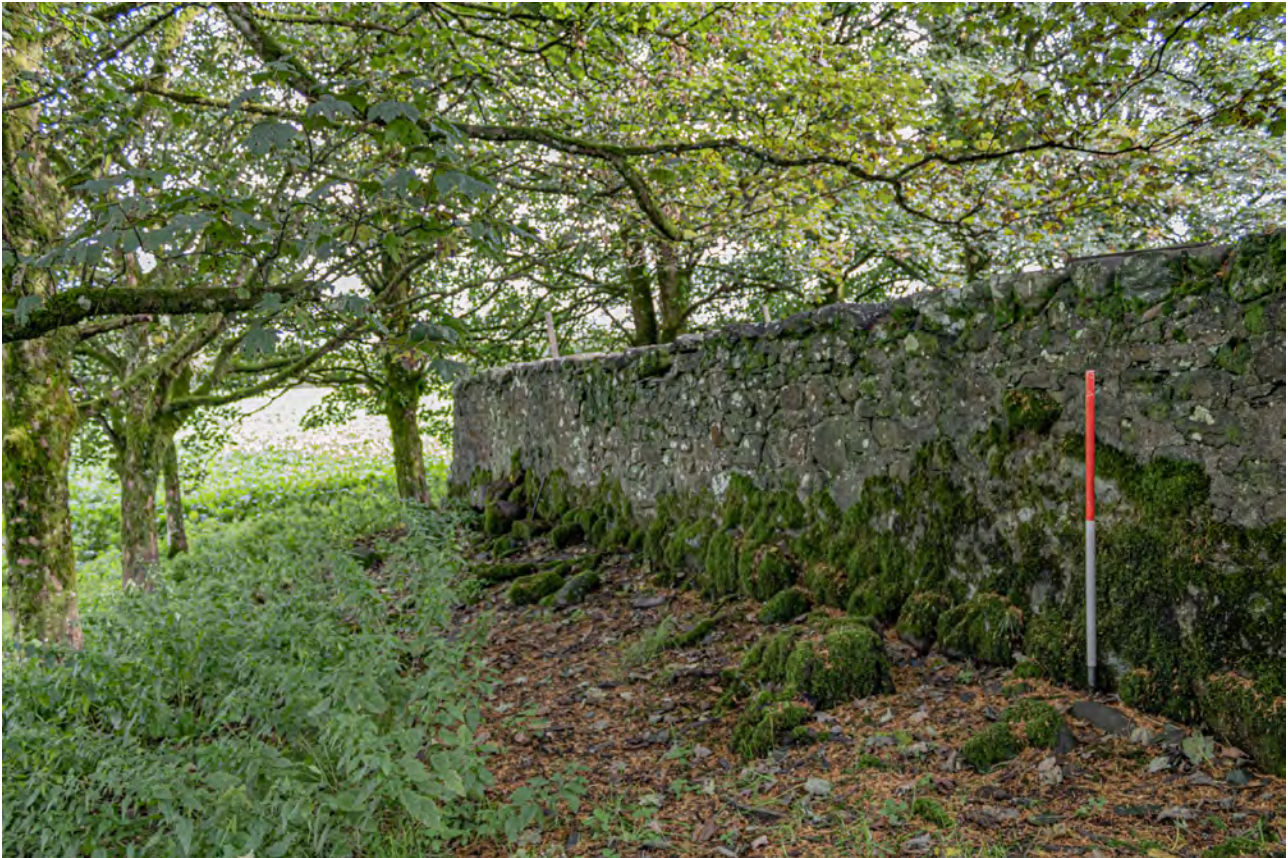
Plate KG2: Kilmahog Graveyard, east boundary wall, general view from the north-east
