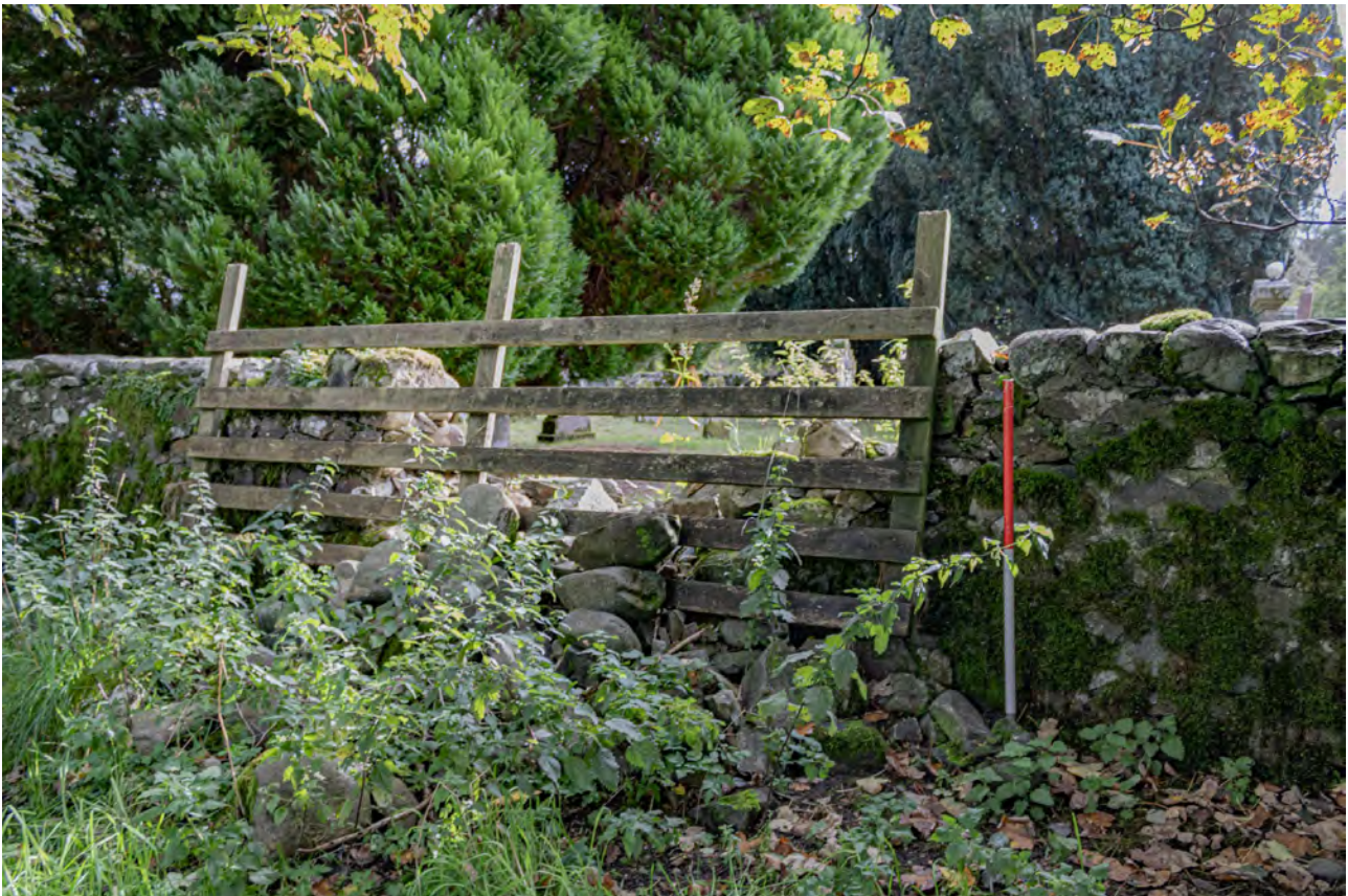
Plate KG11: Kilmahog Graveyard, north boundary wall, detail of damage from the north
