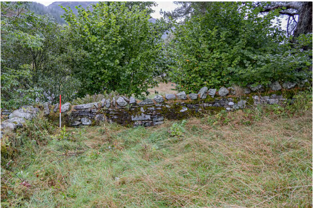
Plate SB4: Saint Bride's Chapel, north enclosure wall, general view from the south
