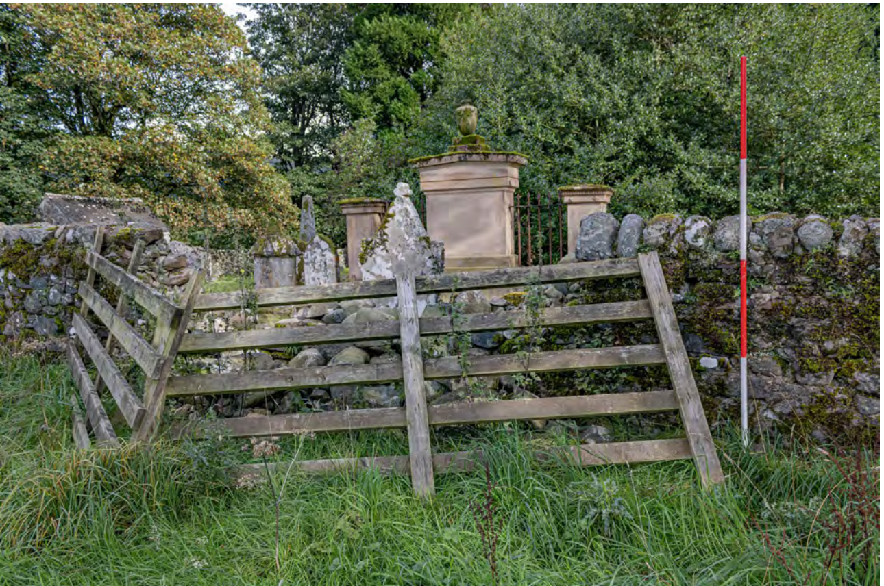
Plate KG15: Kilmahog Graveyard, west boundary wall, detail of damage from the west
