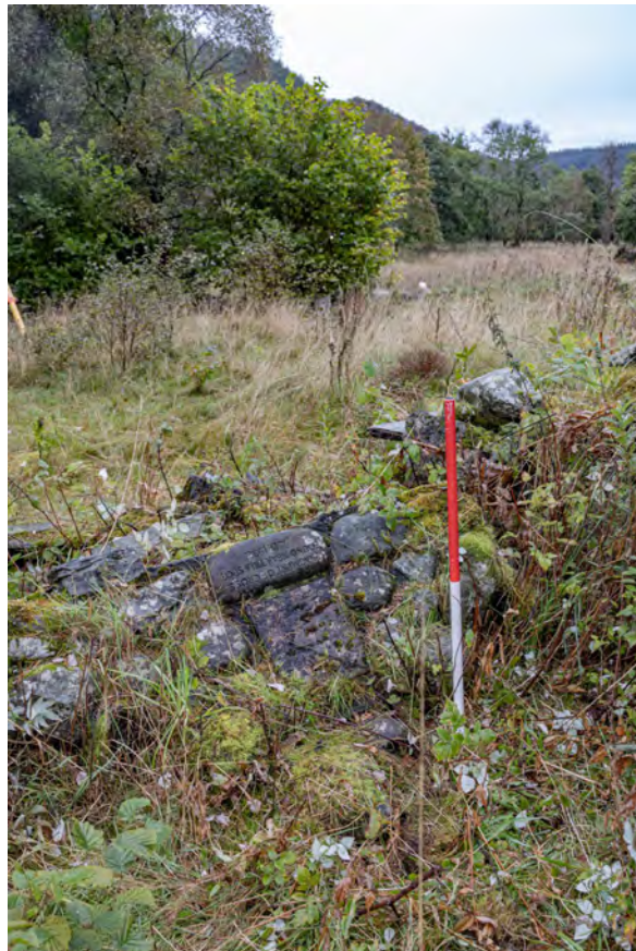
Plate SB8: Saint Bride's Chapel, detail of collapsed section of wall from the north
