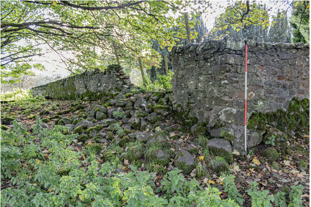
Plate KG12: Kilmahog Graveyard, east boundary wall, detail of damage from the north-east
