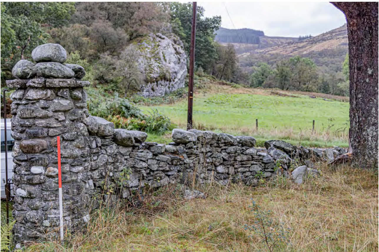
Plate SB6: Saint Bride's Chapel, detail of the gate pier from the west
