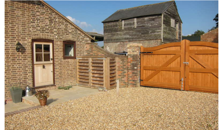
Example of screened air source heat pump
