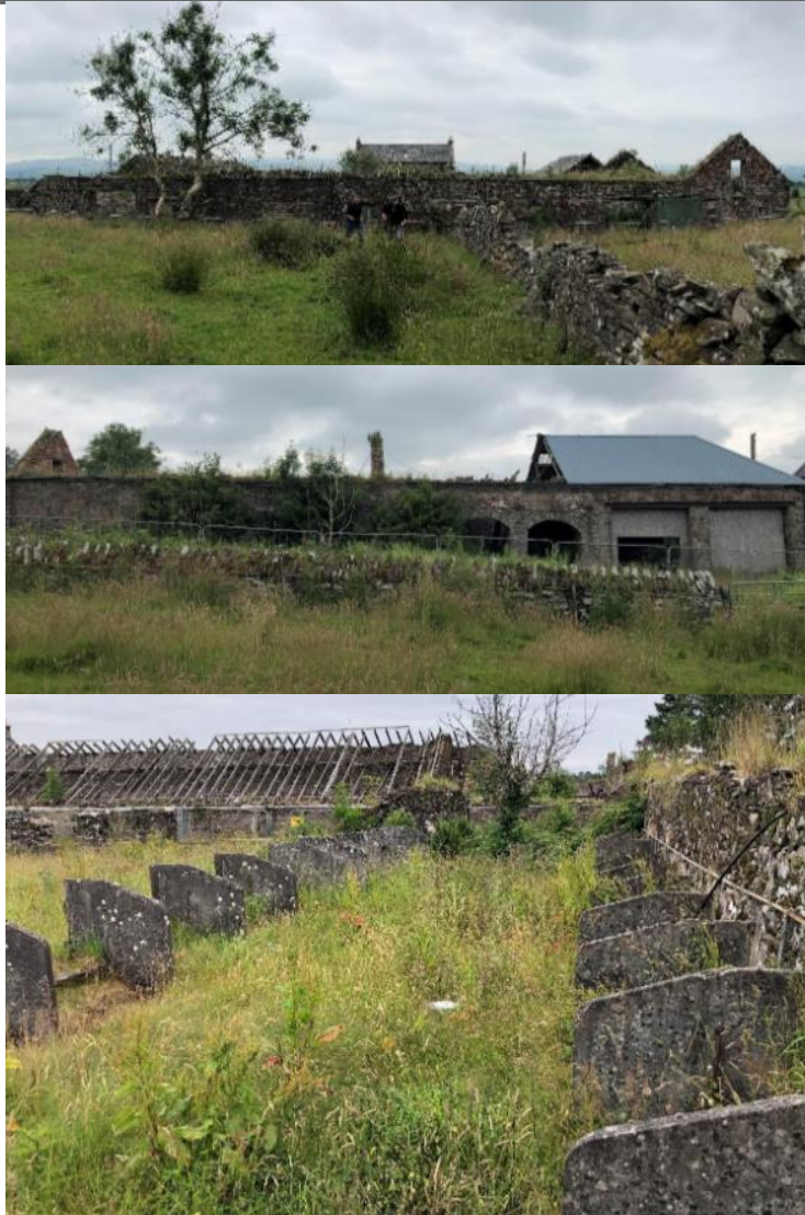
Figure 5: Photos of the existing steading building - photos (in sequence from top to bottom) of north-eastern corner of steading; north-western corner; north elevation; west elevation; and former cattle stalls to the east of the steading.
