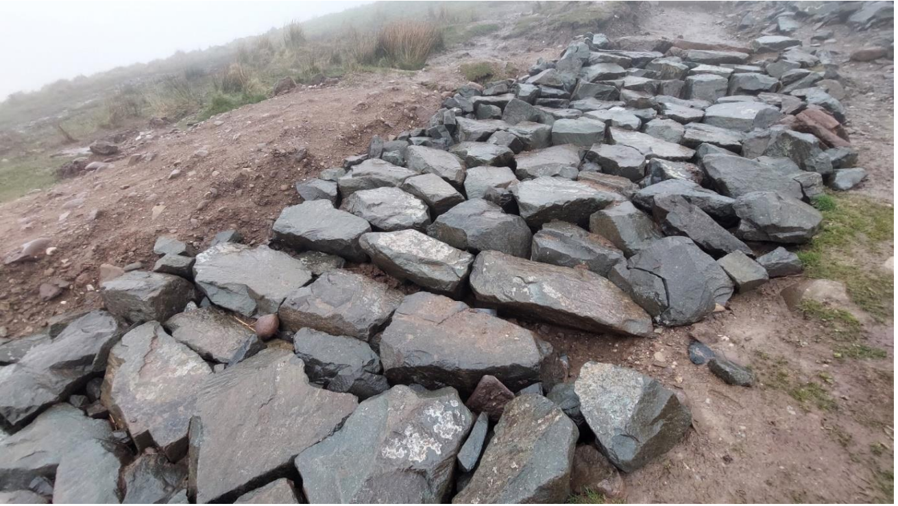
Photo 2: Large gaps between stones, April 2024
